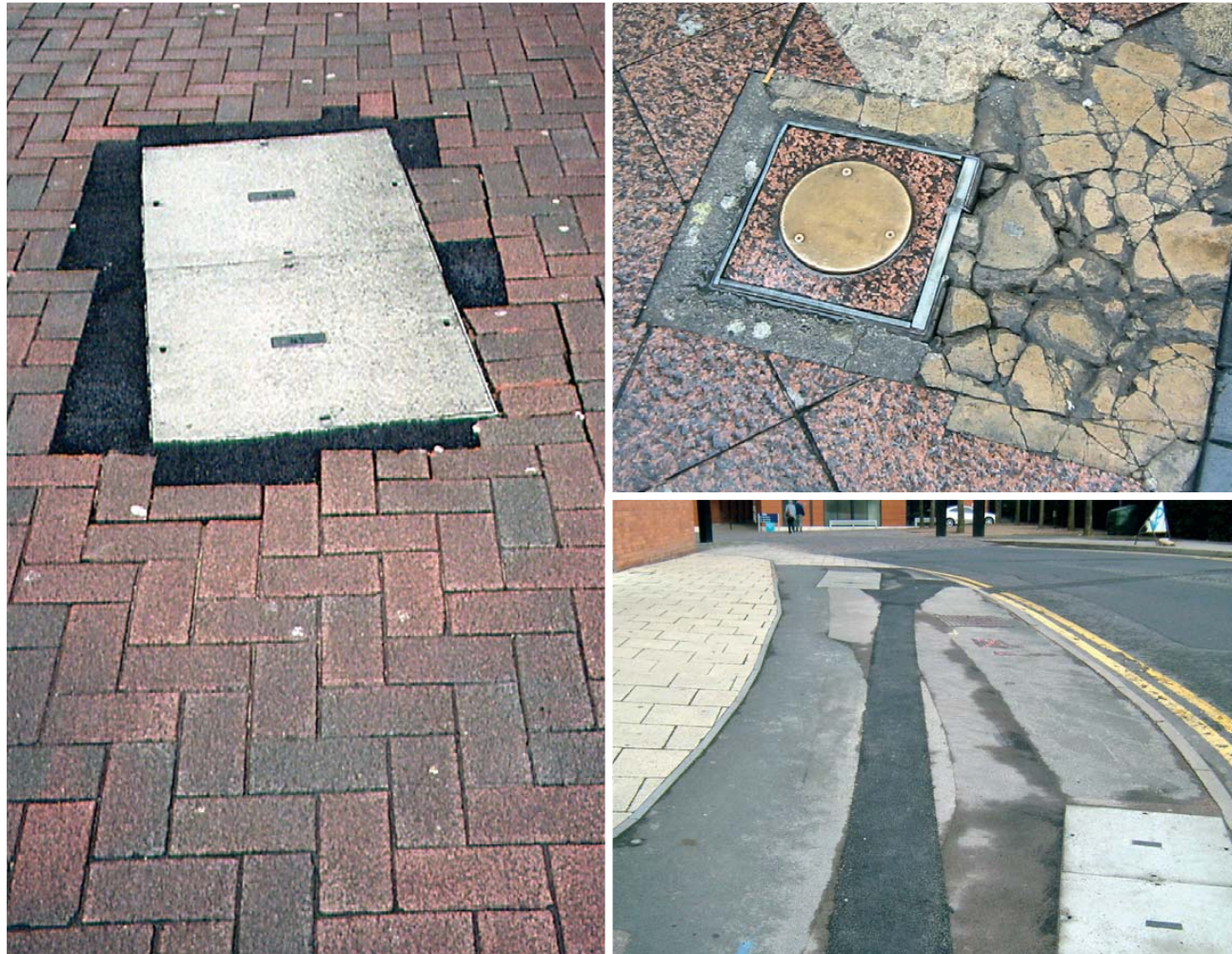
Fig 9.1 poor choice of materials and poor maintenance can damage the character of any area
